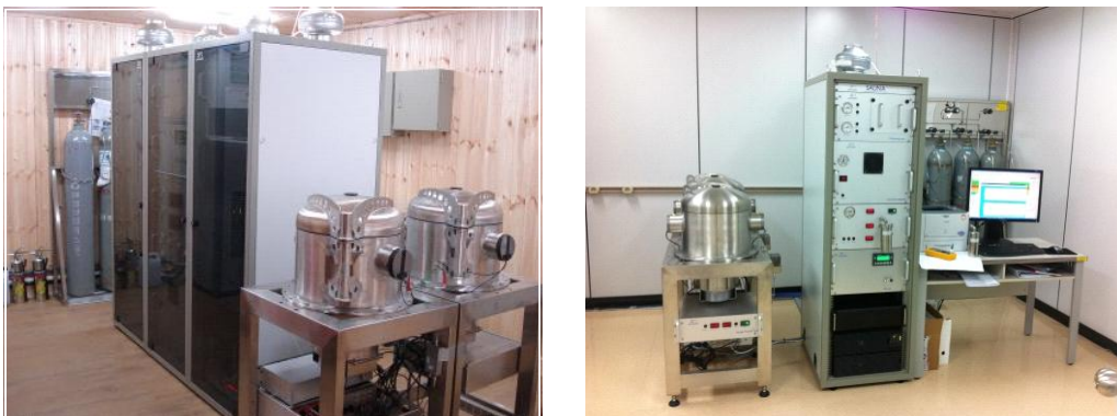
Fig. 5.1 Fixed radioactive Xe monitoring system(SAUNA II-IMS) and analyzer for mobile sampler(SAUNA II-Lab)
